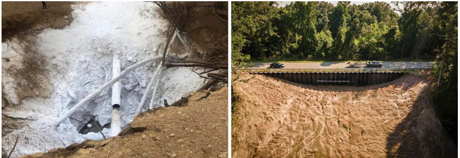
LEFT: The CO2 pipeline rupture. RIGHT: Vehicles pass over the pipeline explosion site in Satartia in July. Yazoo County Emergency Management Agency/Rory Doyle for HuffPost
